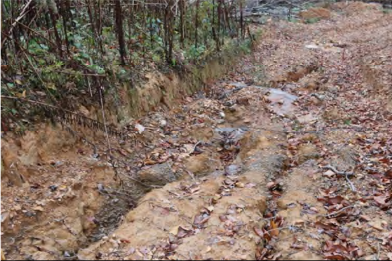
59 Little Cedar Stands, LLC 35.513923 -87.895415 03-NOV-17 5:50:55PM SE 649' 2' gulley in skid trail, steep slopes
