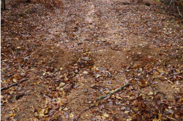
35 Little Cedar Stands, LLC 35.514792 -87.907041 03-NOV-17 2:01:18PM S 643 Water bar eroded through
